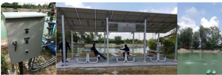
Solar power Motor Generator for Classroom, lighting, Pumping system
