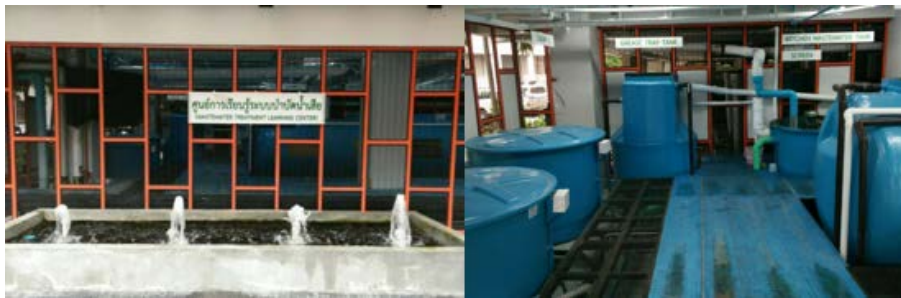
Wastewater treatment from the main cafeteria in Bangkok campus
