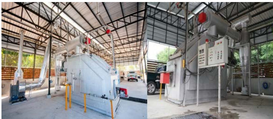
Combine Heat and Power from the Eco-Friendly Waste Incinerator
