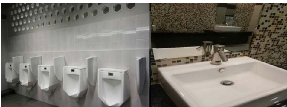
Automated restroom for saving water
