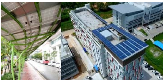
Solar Panel on cover way and rooftop on Faculty of Science, Environment and Energy building
